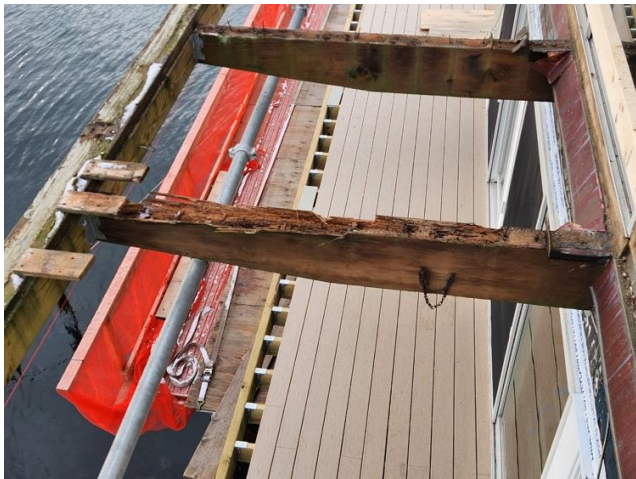
Figure 2 Visible rot on the support beams of the second floor East-facing deck
